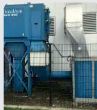
De centrale las- rookafzuiging
